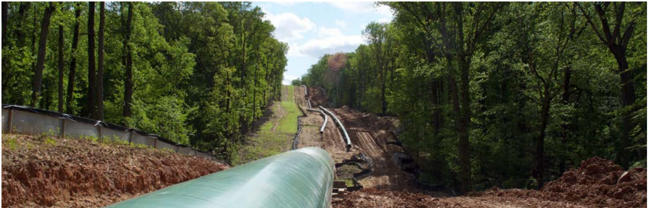
Construction staging area & right-of-way -26" pipeline. Photo credit: Sierra Shamer retrieved from: https://www.frackracker.org/2016/06/introduction-oil-gas-pipelines/
